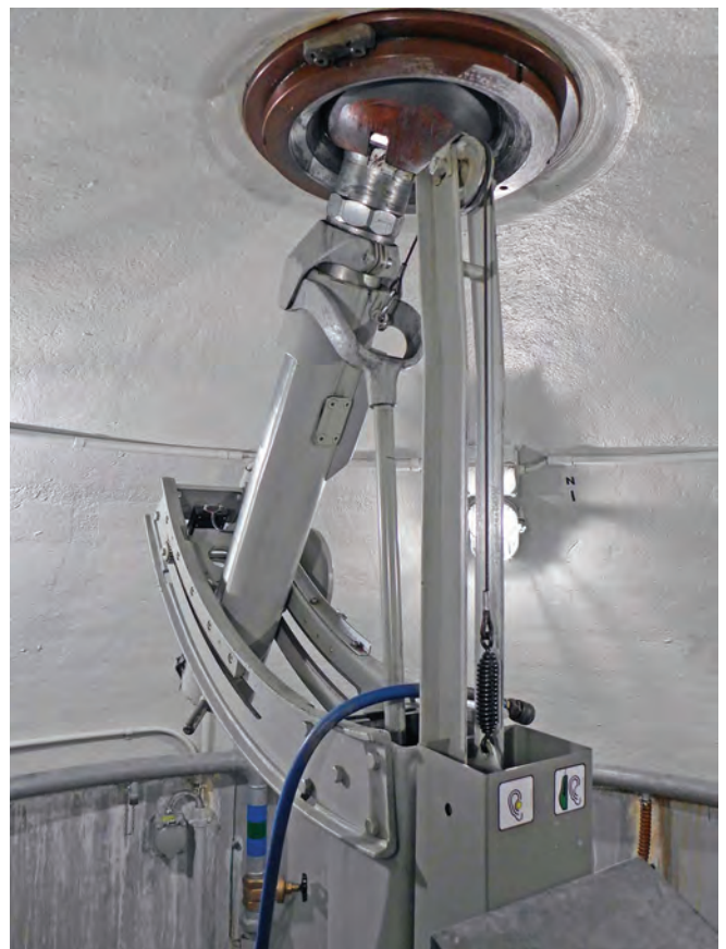
Fort Magletsch: One of the 8.1cm mortars installed in armoured cupolas during the 1960s
